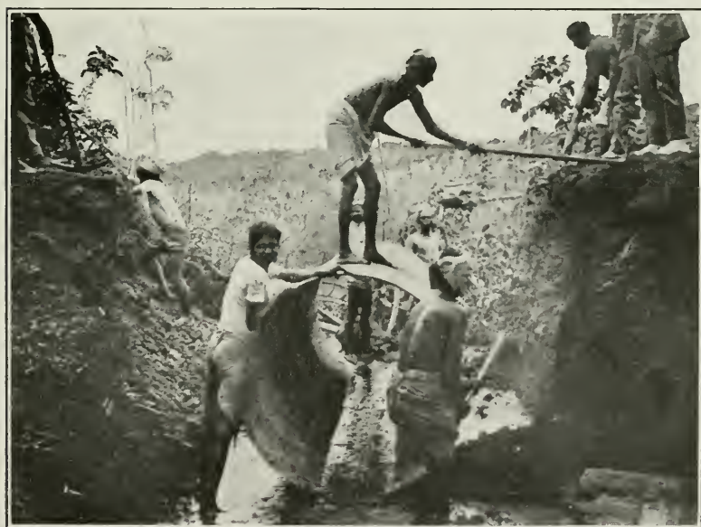
FIG. 13.—An Armeo Culvert in the Malay Peninsula. The American Rolling Mill Company exports rust-resisting products to far corners of the round world.
